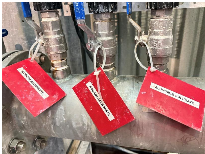
Figure 2 photos of chemical supply at water treatment plant
