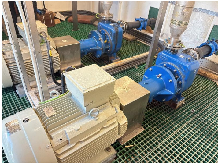
Figure 1 Water pumps at Murrell River Reservoir
